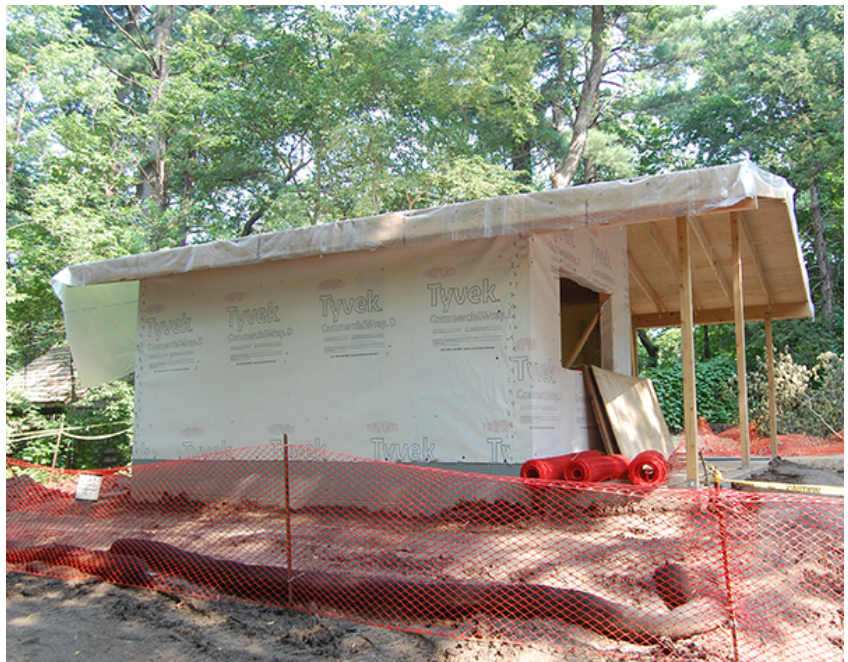
Construction continued into the summer on the storage building at the Garden.
